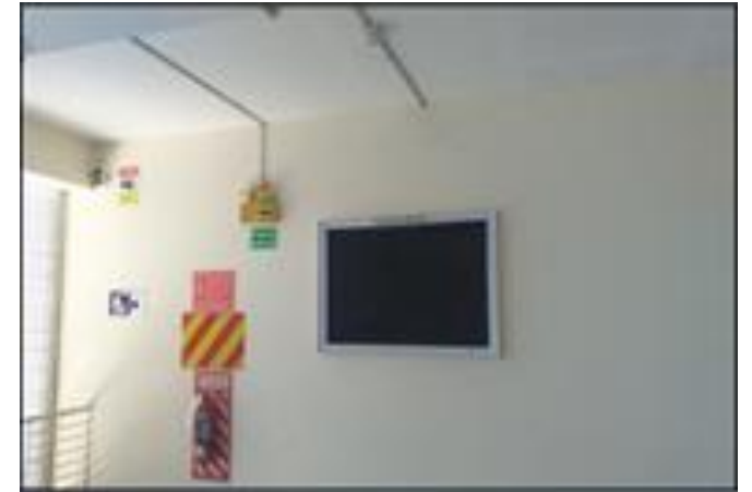
Fire Extinguisher & Smoke Detector
