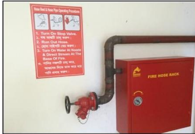
Fire Hose Rack with using Instruction in Every Floor
