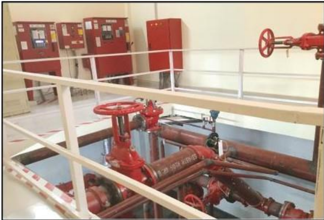
Fire Hydrant System
